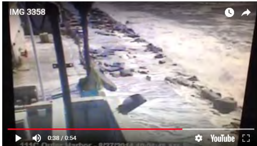
South Swell Damage 8-27-14
