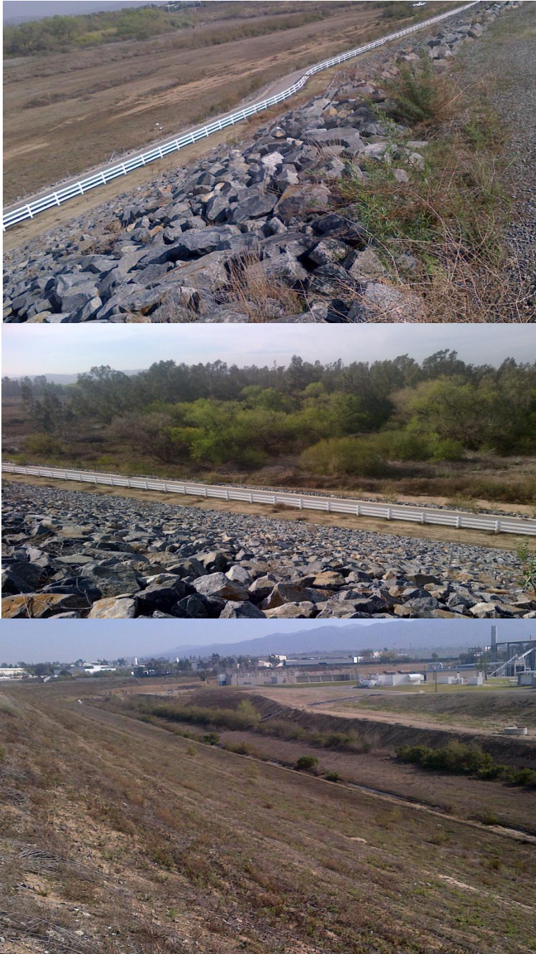
Photo 3 (top) Sewage Treatment Dike facing northeast; Photo 4 (middle) facing northwest toward the reservoir; Photo 5 (lower) depicts the landside of the Sewage Treatment Dike.
